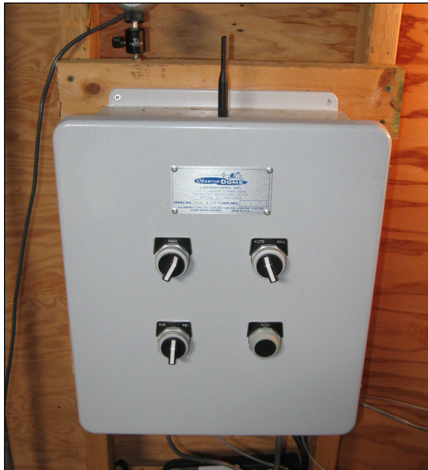
FIG. 31. The dome azimuth control module. (Author)
